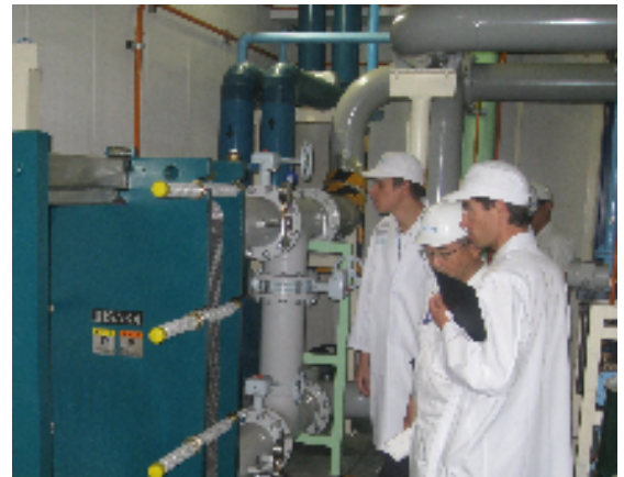
Liquid treatment area at Extra-large Bearing Plant
